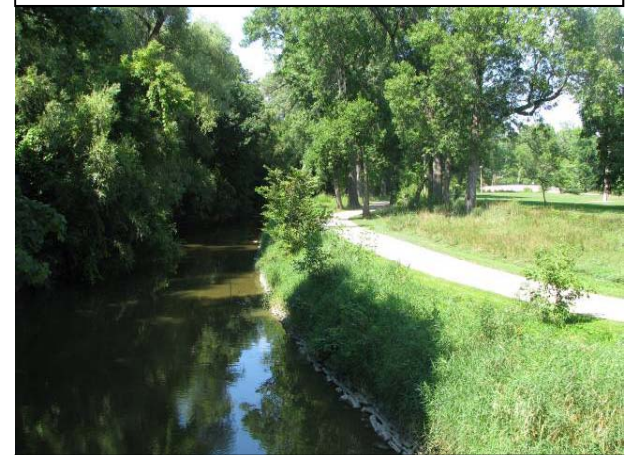
View looking north from footbridge at east bank. Conditions = high grass and little sign of erosion.
