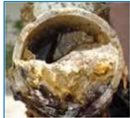
Sewer pipe clogged with grease
